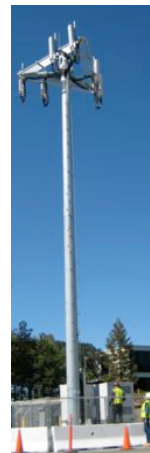
Figure 2: AT&T Cell Phone Tower at SLAC
