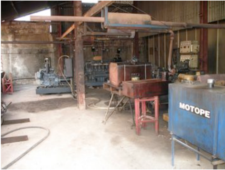
Figure 2: A building housing generators for an ISP in Guinea Bissau. The closest generator was poorly tuned and exhausted into the room, causing dangerous levels of carbon monoxide to accumulate in the work area.
