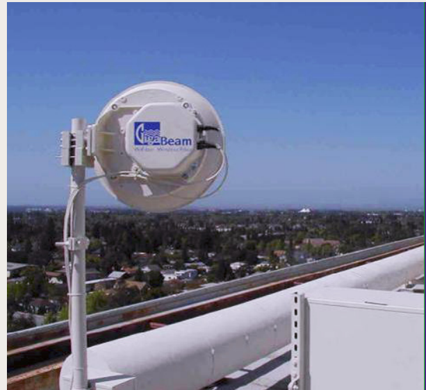
Figure 11: GigaBeam installation providing backhaul for Google's Mountain View Wi-Fi Network
